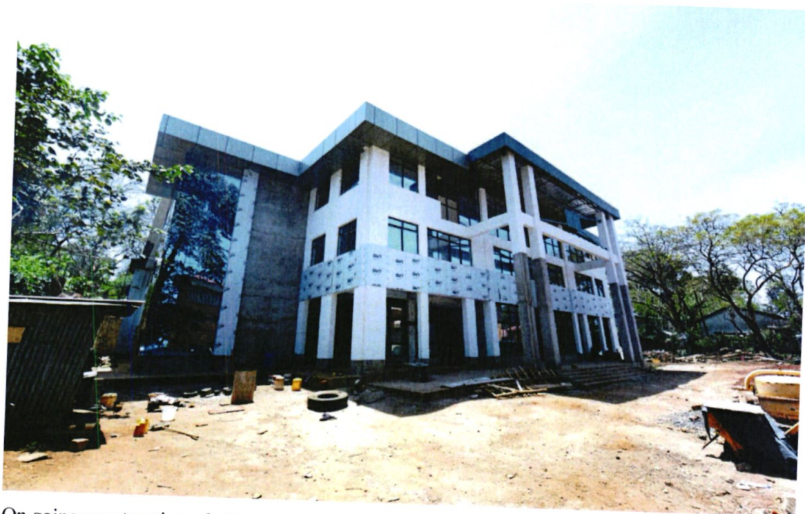
On going construction of ultra-modern chamber for the County Assembly of Marsabit.
