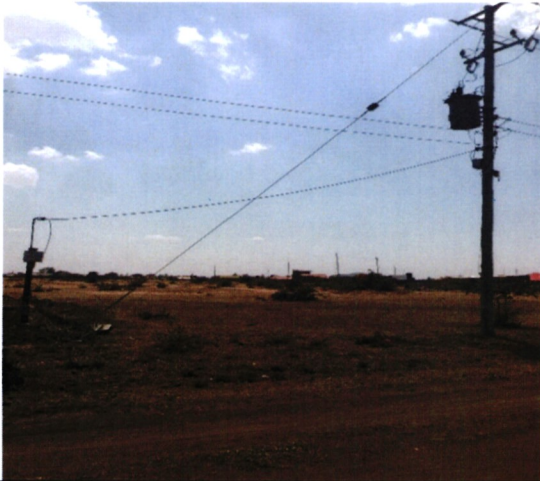
Picture 3: Service cables erected on parcels of land with non-existing households at Langata estate, Kiambu County
