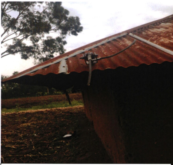
Picture 1: Vandalized service cable at Mariri Primary School, Homabay County
