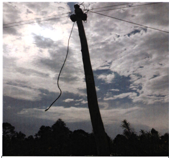
Picture 2: Vandalized protective multiple earthing at Madenge Shopping Centre, Kakamega County
