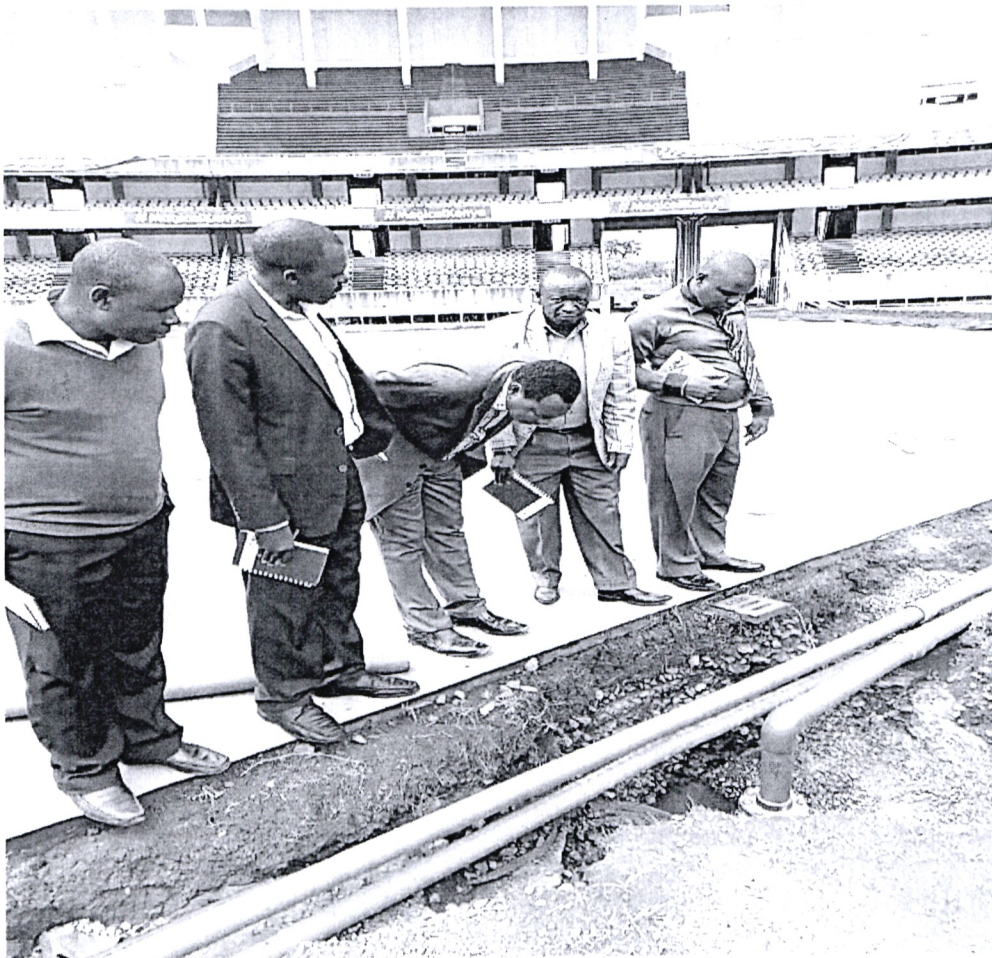
Figure 21: Effects of heavy rains on ongoing Projects
