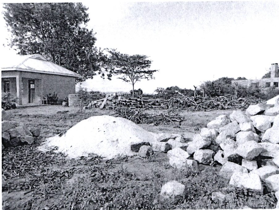
Figure 14: various materials including borehole drilling pipes and perimeter wall stones on site but not well stored
