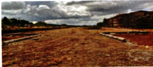
CIVIL WORKS DRIVEWAY & PARKING COMPACTED SURFACE READY TO RECEIVE CABBRO BED AND CABBRO SURFACE FINISH
