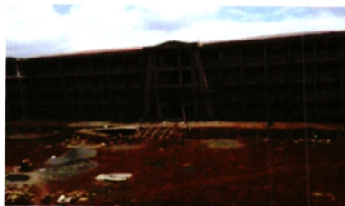
CIVIL WORKS COURT YARD RAMP AND STAIR CONSTRUCTION TO ENTRANCE BLOCK A
