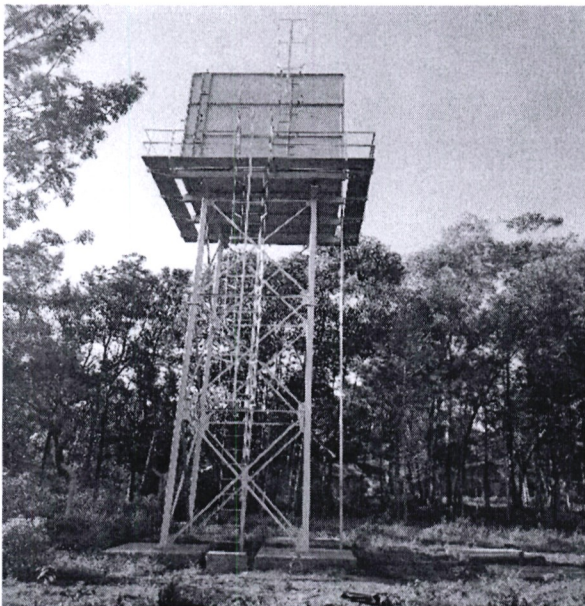
Photo: 3X3 M 3 Water tank for water supply
