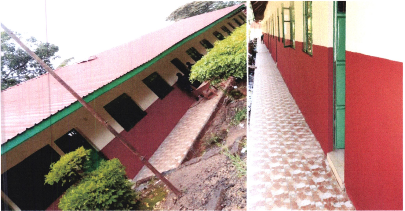
MBIRI PRIMARY SCHOOL CLASSROOMS AT TOWNSHIP WARD AFTER RENOVATION BY KIHARU NG-CDF
