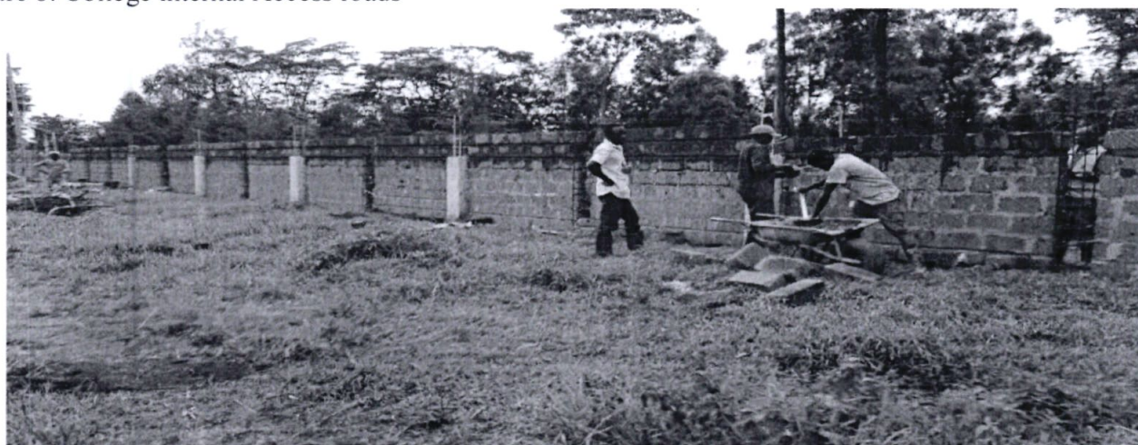
Figure 9: Construction of the College Perimeter wall to enhance security and safety of its property at Ksh 250M.
