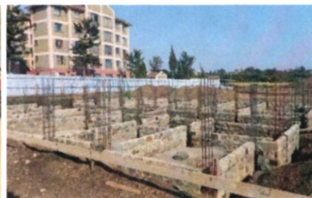
The ongoing works at the Kanyakwar Phase III project in Kisumu Town.
