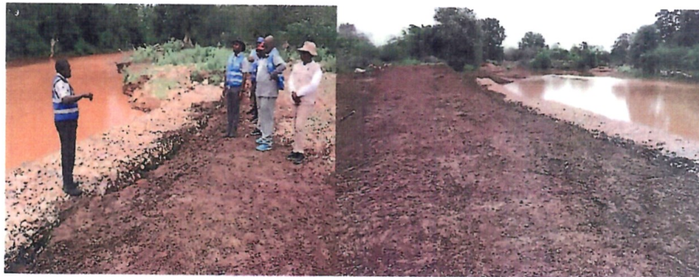
TARDA Chair and MD at the Completed Gabion Protection Works at Kelona (April 2025)
