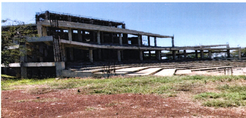
Picture 1: Stalled Construction of the Africities Convention Centre in Kisumu County
