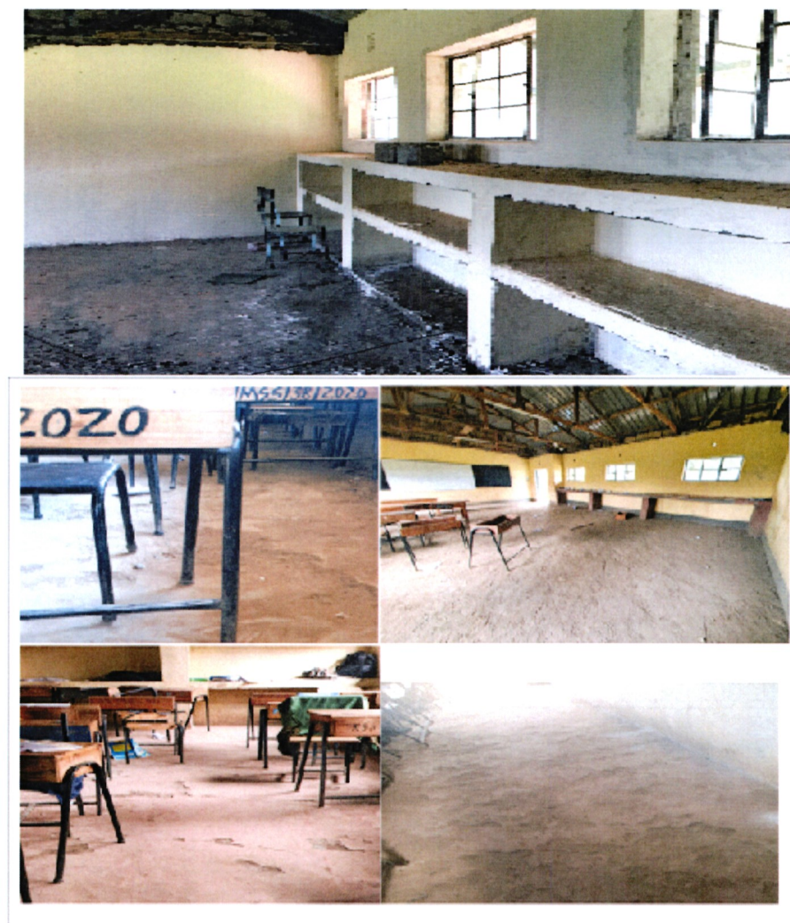
Picture 4: Classrooms with Poorly Constructed Floors
