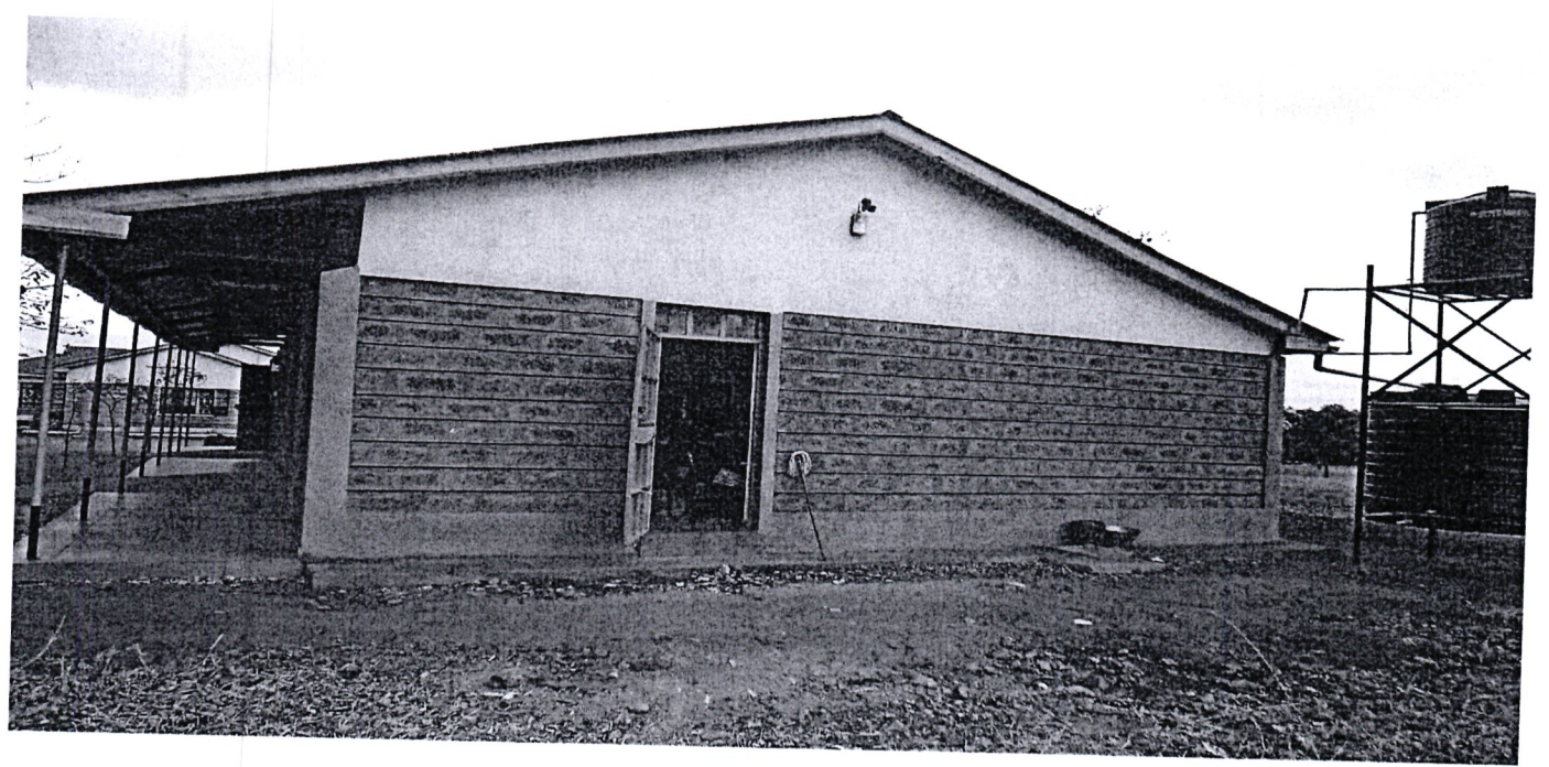
NGUUMO GIRLS SECONDARY SCHOOL-Construction of a science laboratory, supply of 40 stools and 10,000 litres water tank.
