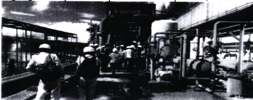
Olkaria I rehabilitation power plant
