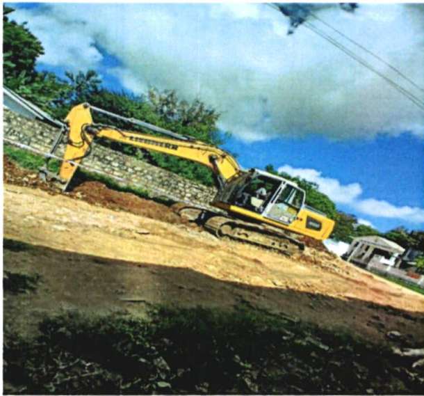
Sub-Surface Drain In Likoni
