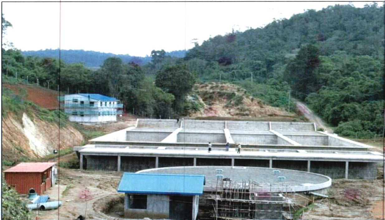
Chemususu Phase II Water Supply & Distribution Project Treatment Plant Component
