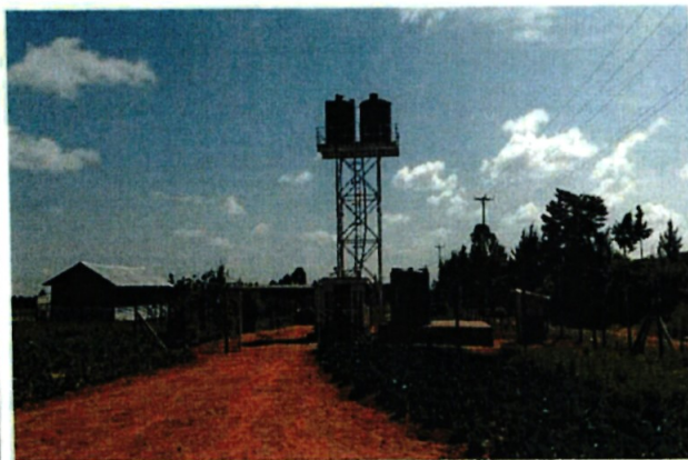
Borehole, water harvesting & storage in Laikipia
