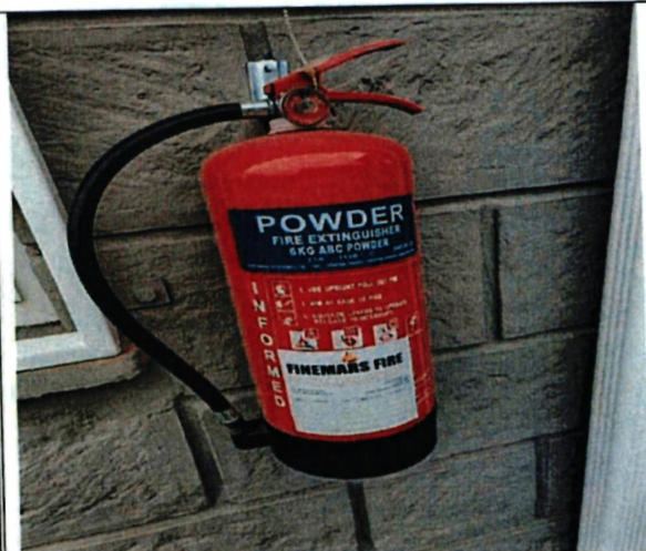
Fire extinguisher in Makueni farm for fire safety
