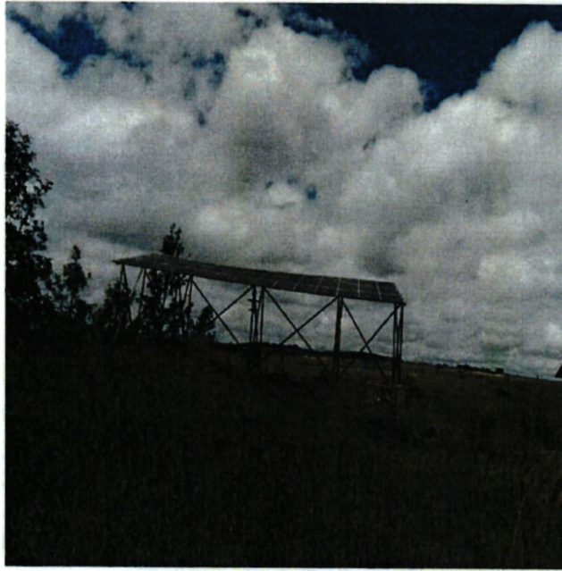
Solar Power water pumping system in Narok
