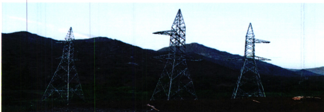
Loop in Loop Out (LILo) towers at Ortum substation of 138km 220kV Turkwel – Ortum – Kitale project
