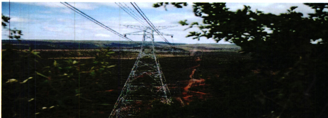
Special tower along 103km 400kV Suswa - Isinya project
