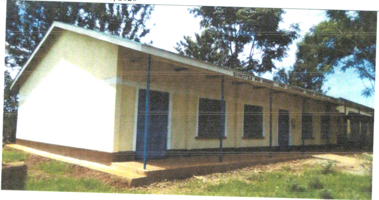
Shirotsa Primary School - Construction of 2no. classrooms to completion. Located in Kisa West Ward. Costed Ksh.1,700,000.
