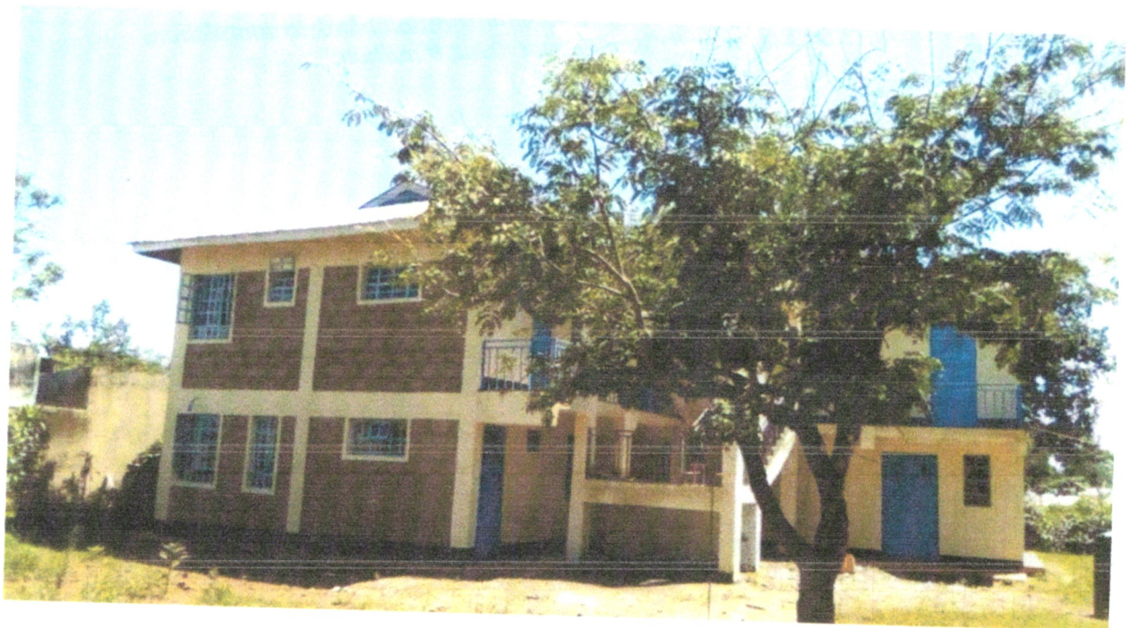
Khwisero West Division, ACC's offices constructed. At finishing level. This is a security project and the first one of its kind in the constituency. It is costing about Ksh.9.0 million.
