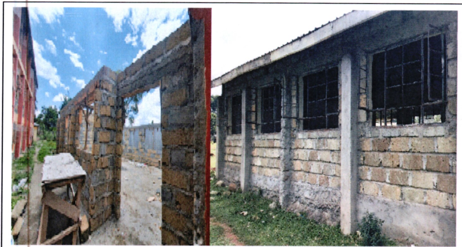
Picture 5 : Incomplete Classrooms
