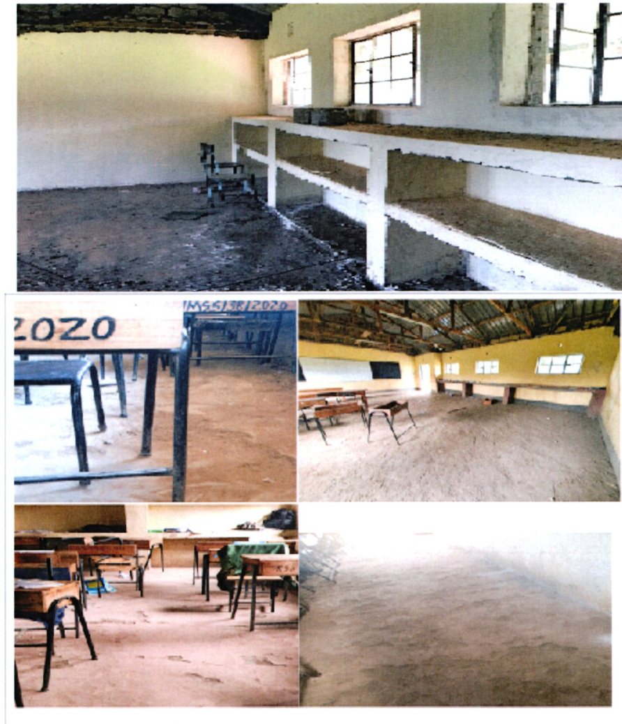
Picture 4: Classrooms with Poorly Constructed Floors
