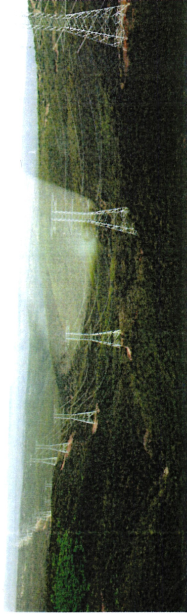
400kV Loiyangalani - Suswa transmission line
