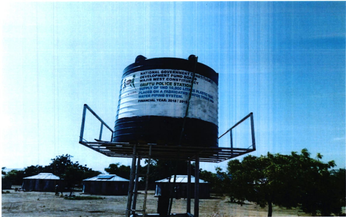
Water piping system at Griftu Police Station, Wajir West Constituency implemented during the FY 2019/2020.
