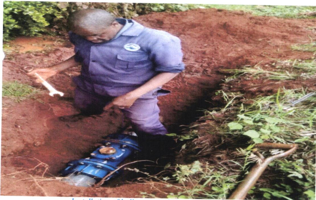
Installation of bulk meter to help in the computation of NRW
