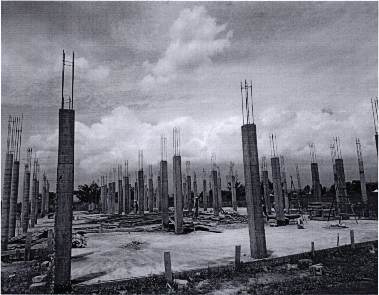
The on-going construction of lecture halls and Administration block at John Okwanyo TTI.
