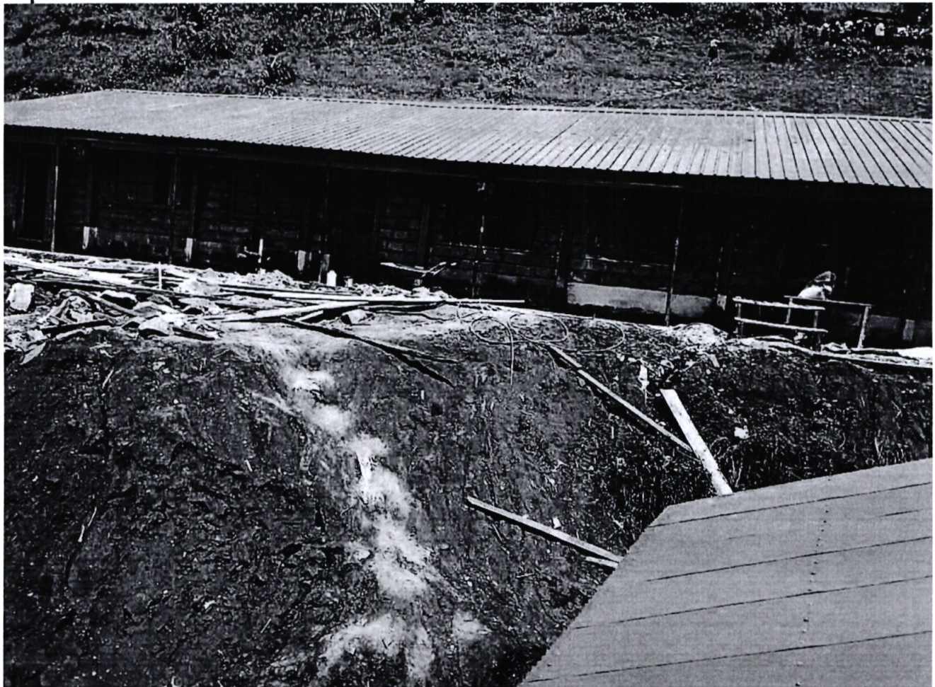
St. Alexander Chongis Mixed Secondary School. Ongoing Construction of three classroom Pokot South NG-CDF has implementation challenges which include;
