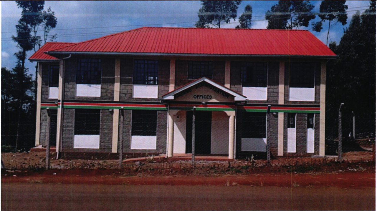
Construction of 7 number Mukurwe Chiefs office (The project expected to enable administrative and other government extension services to approximate population of 29,243 residents of Mugumoini ward)
