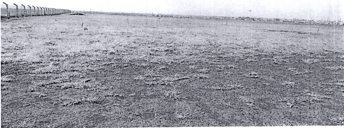
Fig 20: levelling and replanting of grass is complete for Rugby pitch and Football pitch 2. Football pitch 1 is 90 % complete.
