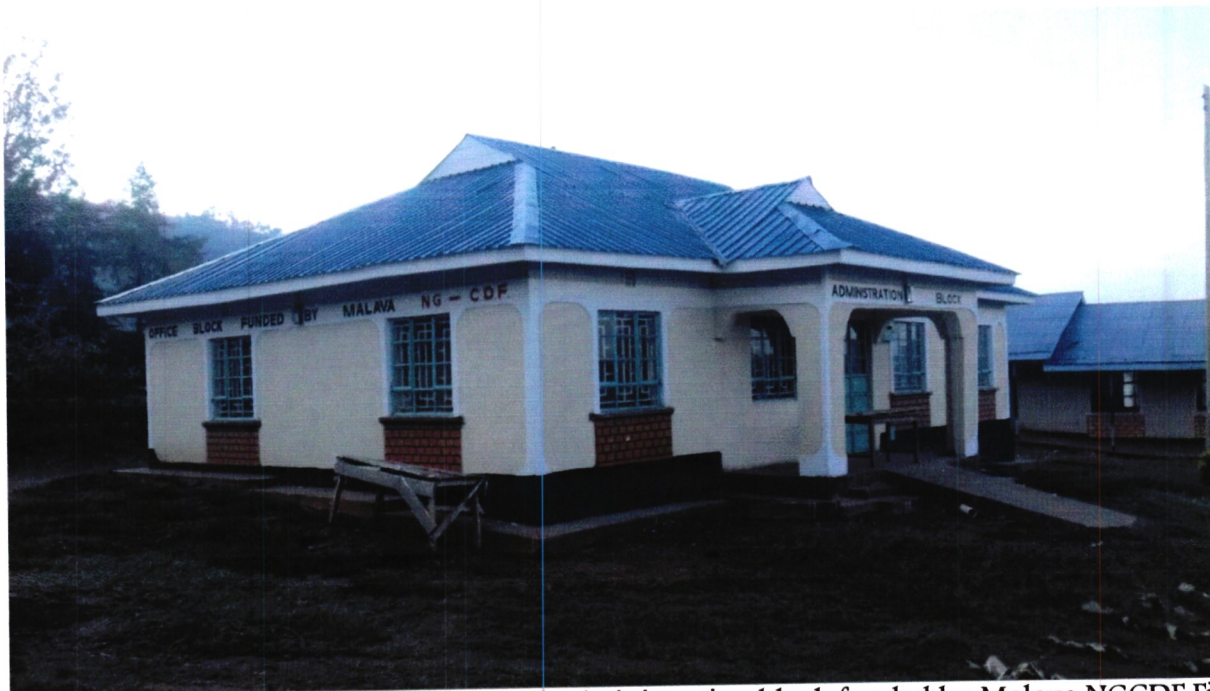
Hamutua Primary School construction of Administration block funded by Malava NGCDF Financial Year 2017/2018
