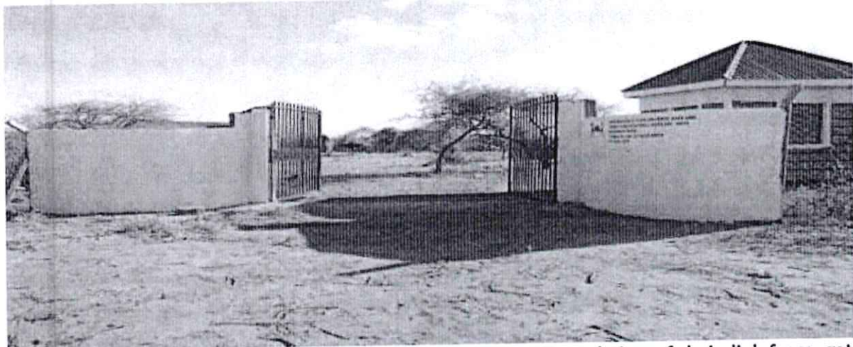
Batalu/Butehelu Mixed Day Boys Sec School: Construction to completion of chain-link fence, gate and guard house
