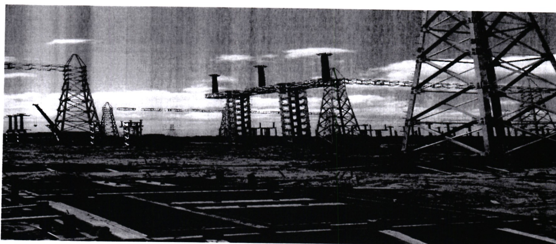
Hvdc Converter Station for 500kV HVDC Eastern Electricity Highway (Kenya-Ethiopia) Project at Suswa
