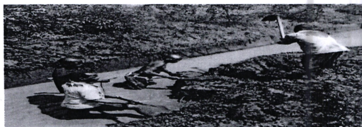
in BM 12-Kimira scheme (Lot 8) O&M - Sections of the main canal identified for clearance and de-silting vs de-siltation of main water conveyance canal in B1 (Kimira Scheme)
