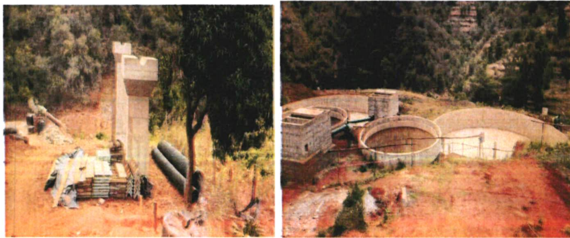
Figure 2: Flying sewerage pipe supporters at Machakos Sewerage project Ongoing Construction of Machakos Sewerage Plant
