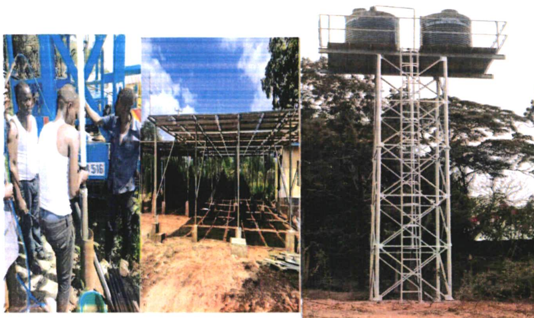
Figure 7: Pump installation and Solar farm for Mwaani Borehole (Wote Water Supply) and elevated tanks for Kitui School for the Mentally Handicapped
