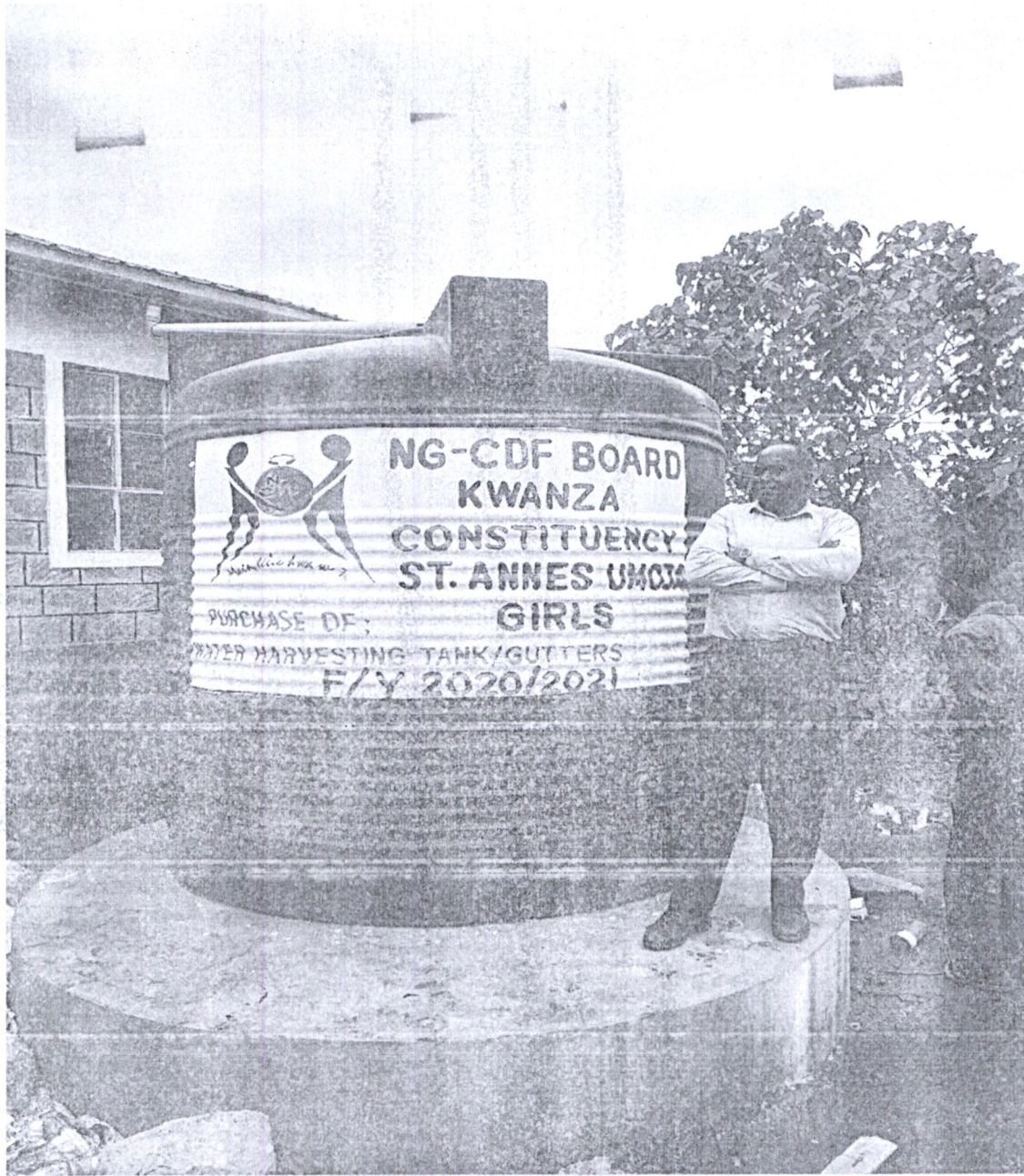
ST ANNES UMOJA GIRLS SECONDARY- PURCHASE AND INSTALLATION OF WATER TANK AND GUTTERS
