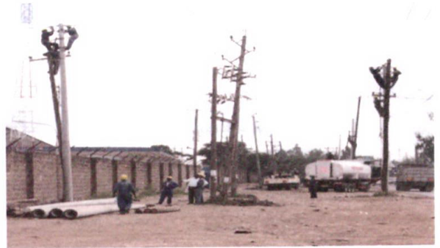
Kenya Power is currently carrying out extensive work on the power infrastructure
