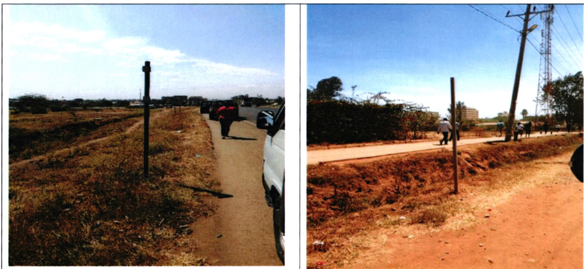
Vandalized road signs along the Eastern By-Pass and Eldoret-Herman Grener Road, respectively. Source: Photos taken by auditors (24 January and 12 February, 2019, respectively).
