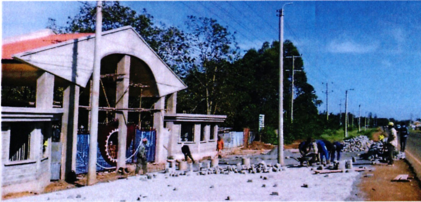
Involvement of the local community and the youth in the construction of The New Main Gate
