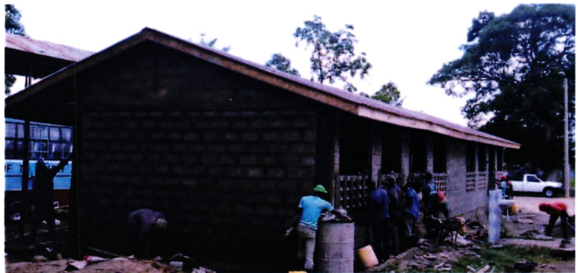
Involvement of the local community and the youth in the construction of Two Number Beauty Therapy and Hair Dressing Classrooms
