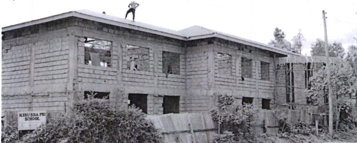
Kiru SDA Primary School: Construction of 12 No classrooms on a 2 storey building.
