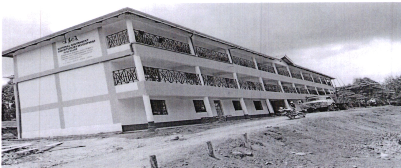
Igorera PAG Comprehensive School: Construction to completion 12 Classrooms On a Storey Building
