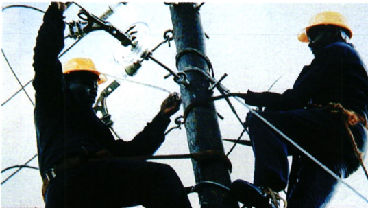
Electricity is transforming life in our rural areas.
