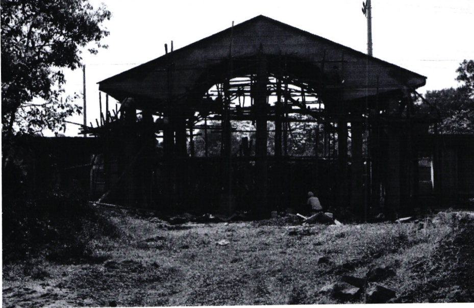
Ongoing construction works of the proposed new gate at Siaya Institute of Technology
