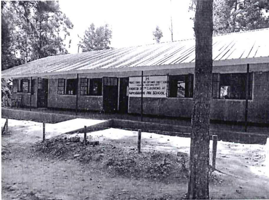
Fig. 3: Kapchemgung Primary School newly renovated 7No. classrooms fully funded by Hamisi NG-CDF 2022/2023 -2023/2024 financial years.
