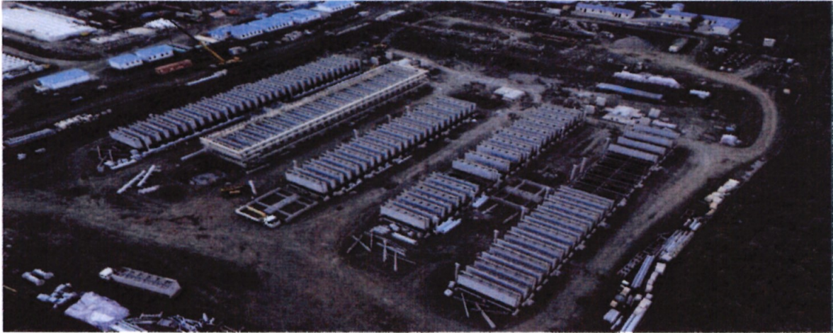
Orpower 22 Power plant as at June 2025
