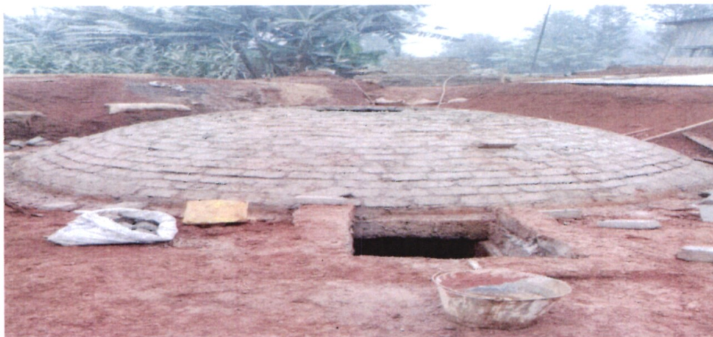
An institutional biogas plant under construction by the State Department for Energy
