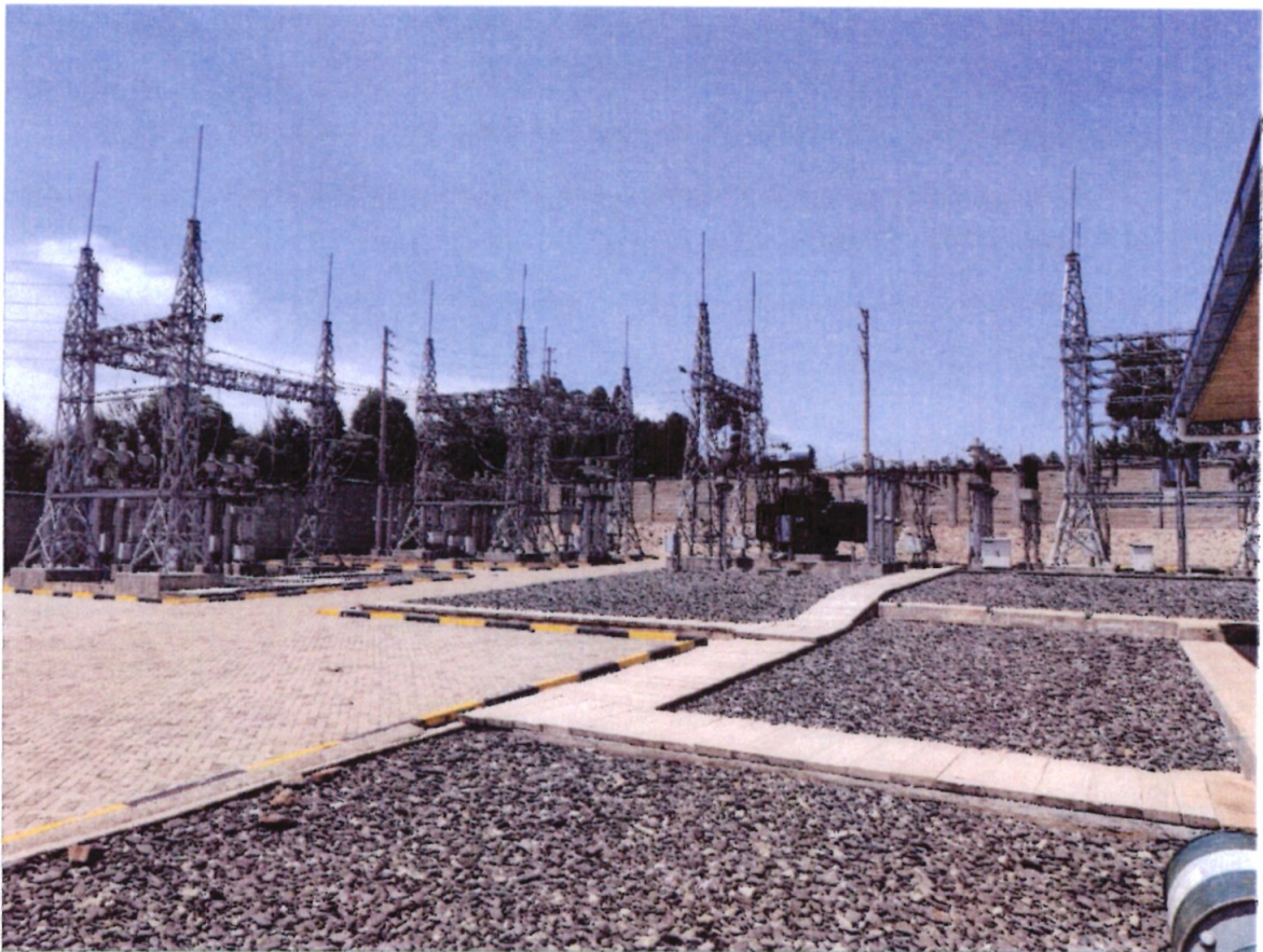
Kabianga Power Distribution substation completed in the FY 2024/2025
