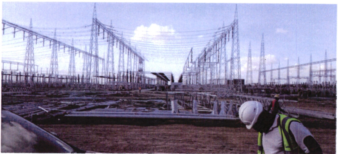
400/220kV Mariakani Substation
