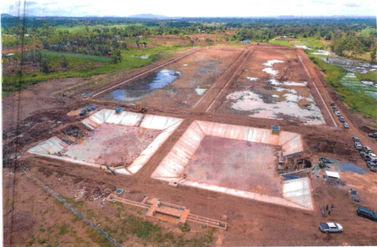
Figure 1: Rwanyange sewerage treatment plant at Meru Sewerage Infrastructure. The sewerage treatment capacity is 8,000M 3 per day.
