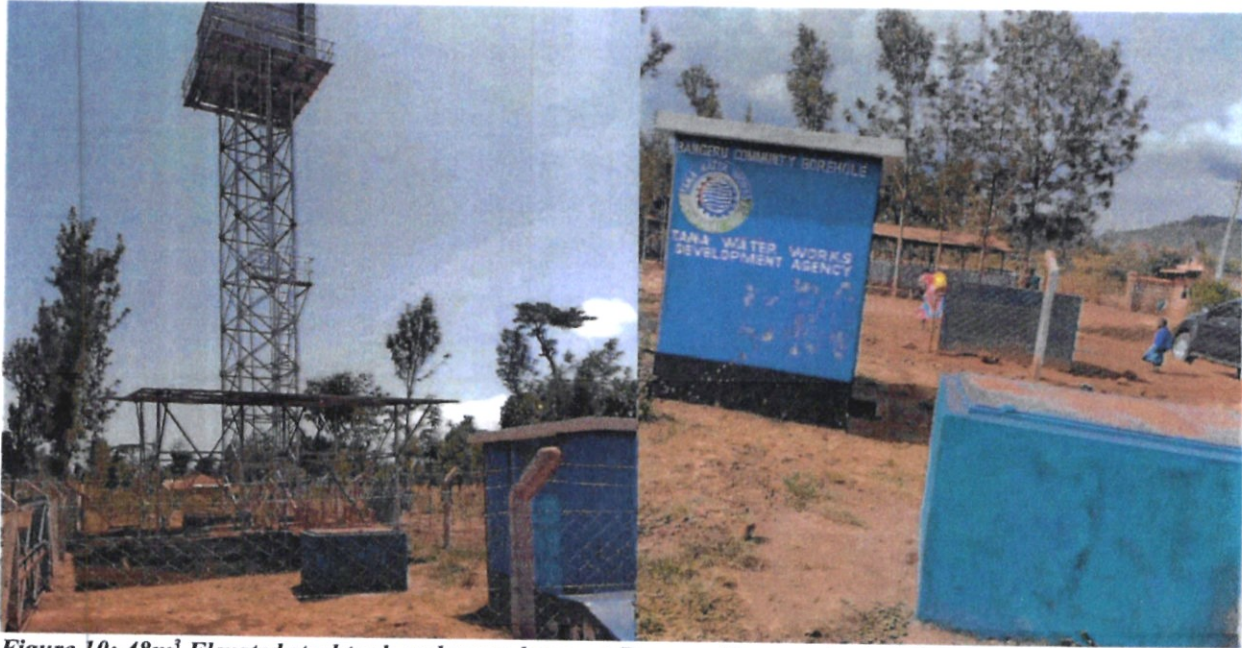
Figure 10: 48m 3 Elevated steel tank and pump house at Bangeru Community Agithi borehole with a yield of 36m 3 /day in Kianjai, Meru County
