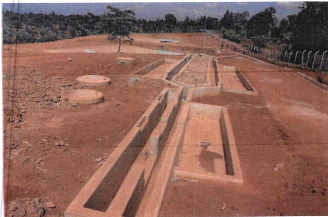
Figure 7: Inlet works at Chogoria Sewerage Infrastructure
