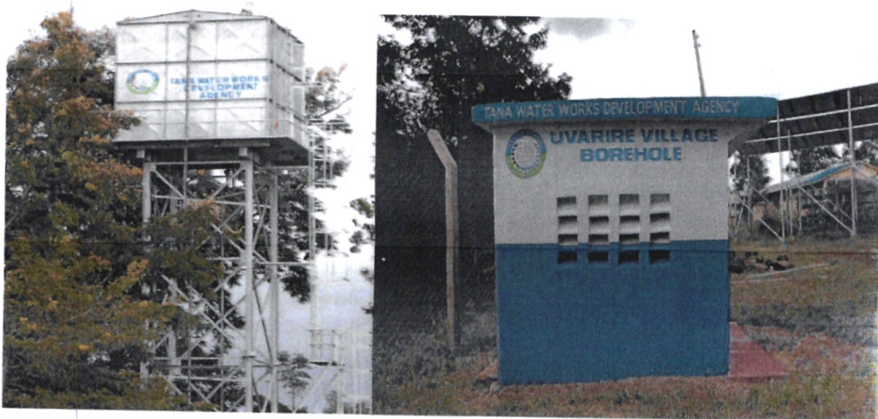
Figure 11: 48m 3 Elevated steel tank and pump house at Uvarire Village borehole with a yield of 12.5m 3 /day in Mbeere, Mbeere Embu County
