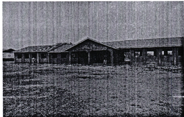
Ongoing project at Ndatani Primary School: Construction of administration block, staffroom and 2No. classrooms
