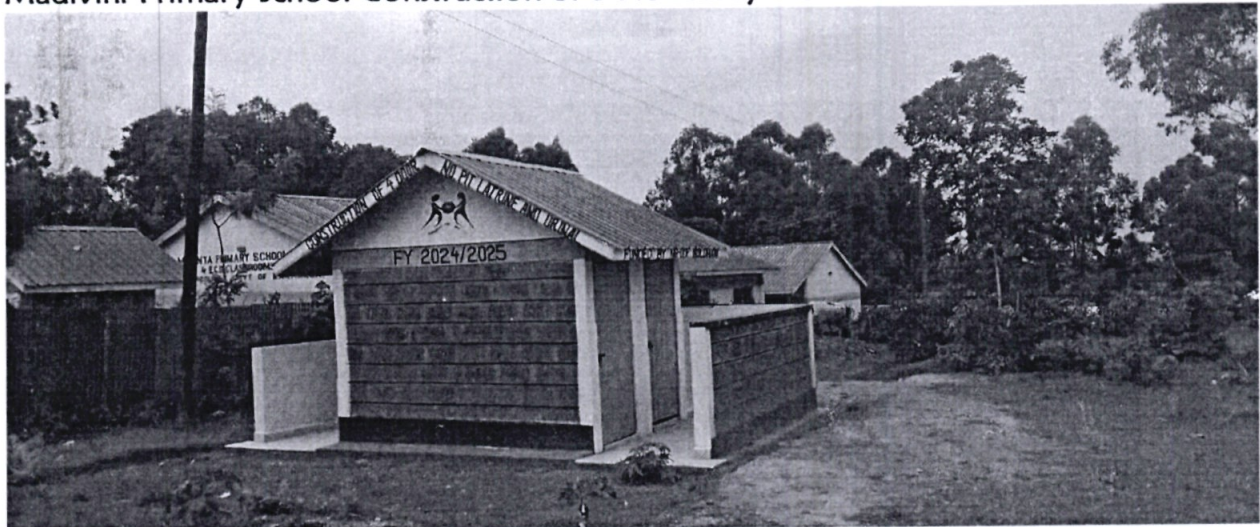
Kakamega South sub-county Education Office -Construction of 4 Door Pit Latrines and Urinal.
