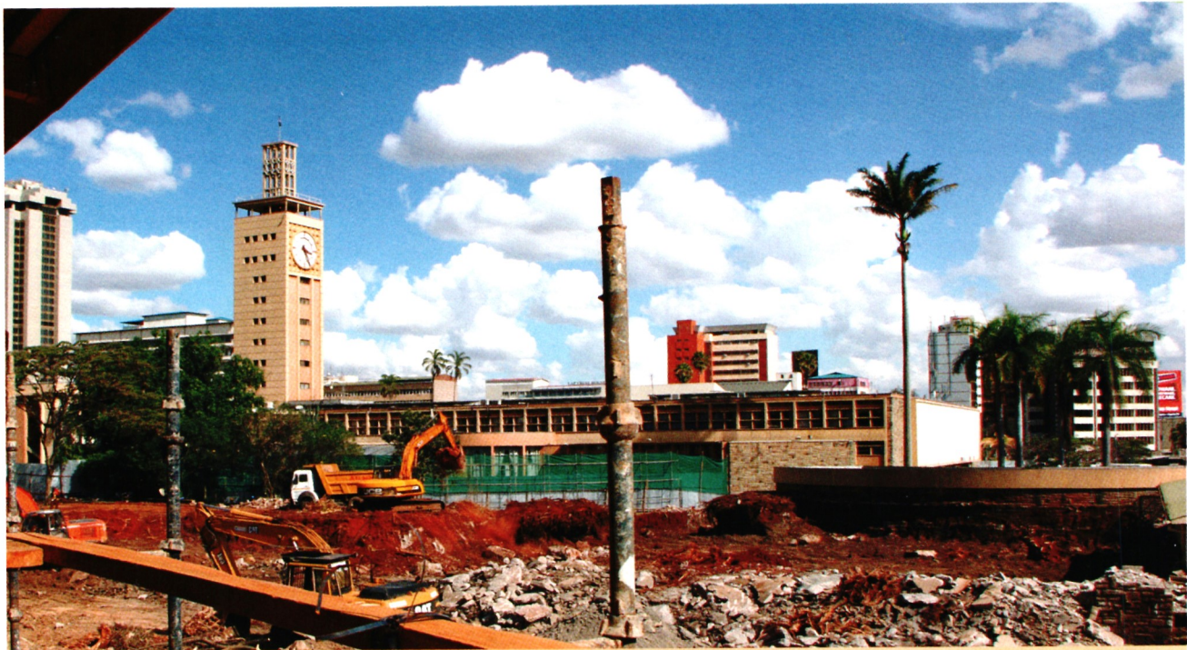
Renovations and construction works at Parliament Buildings to provide accommodation and facilities for MPs
