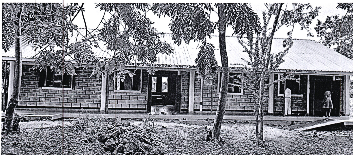
Construction of two (2No.) new classrooms to completion at Bulagu primary school FY – 2021/2022
