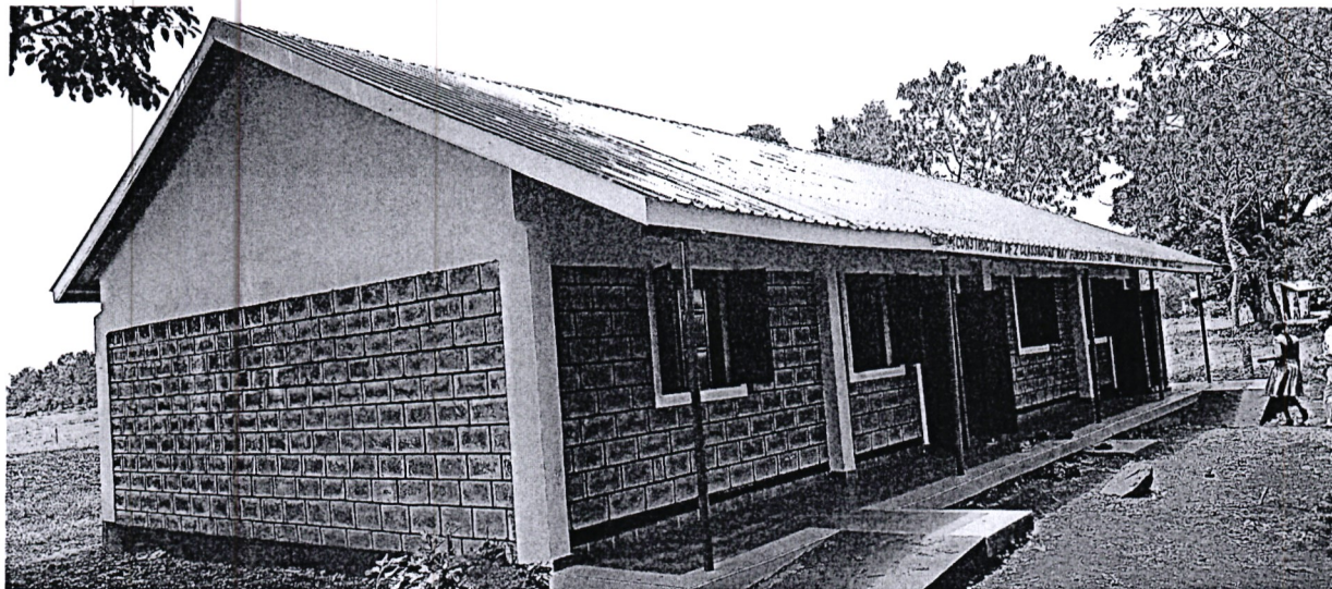
Construction of two (2No.) new classrooms to completion at Bulagu primary school FY – 2021/2022
