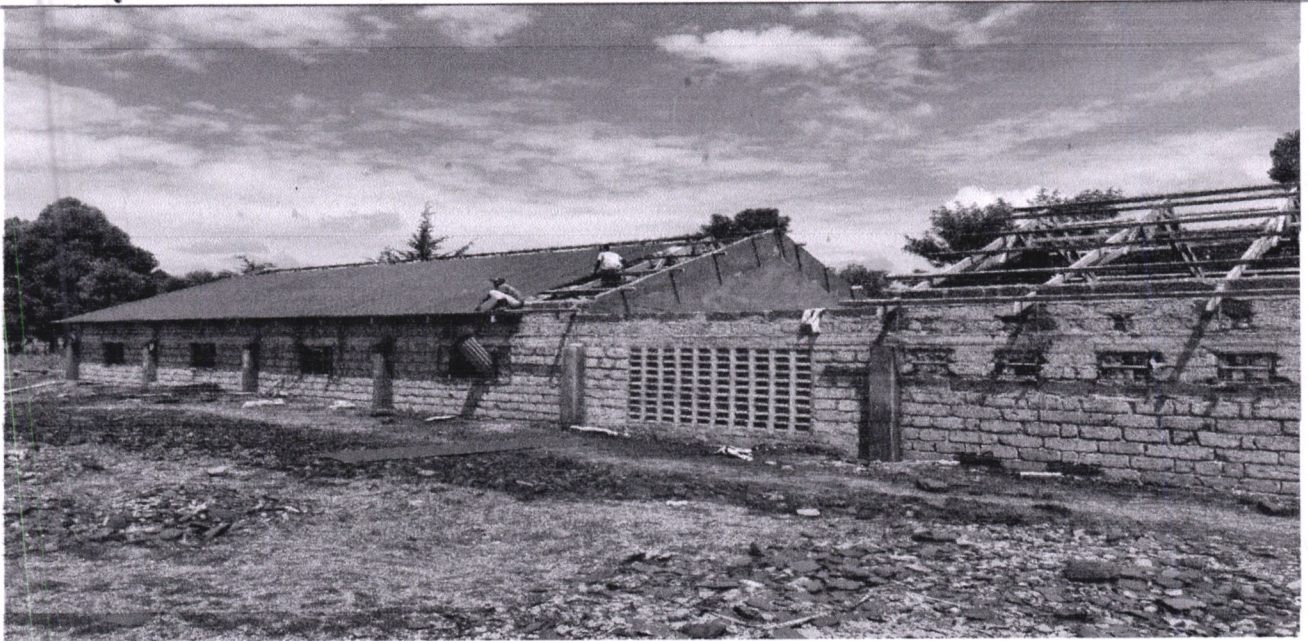
OLASHAPANI BOARDING PRIMARY SCHOOL-96 CAPACITY DORMITORY FUNDED BY NAROK SOUTH NGCDF 2019/2020 (CONSTRUCTION ONGOING)
