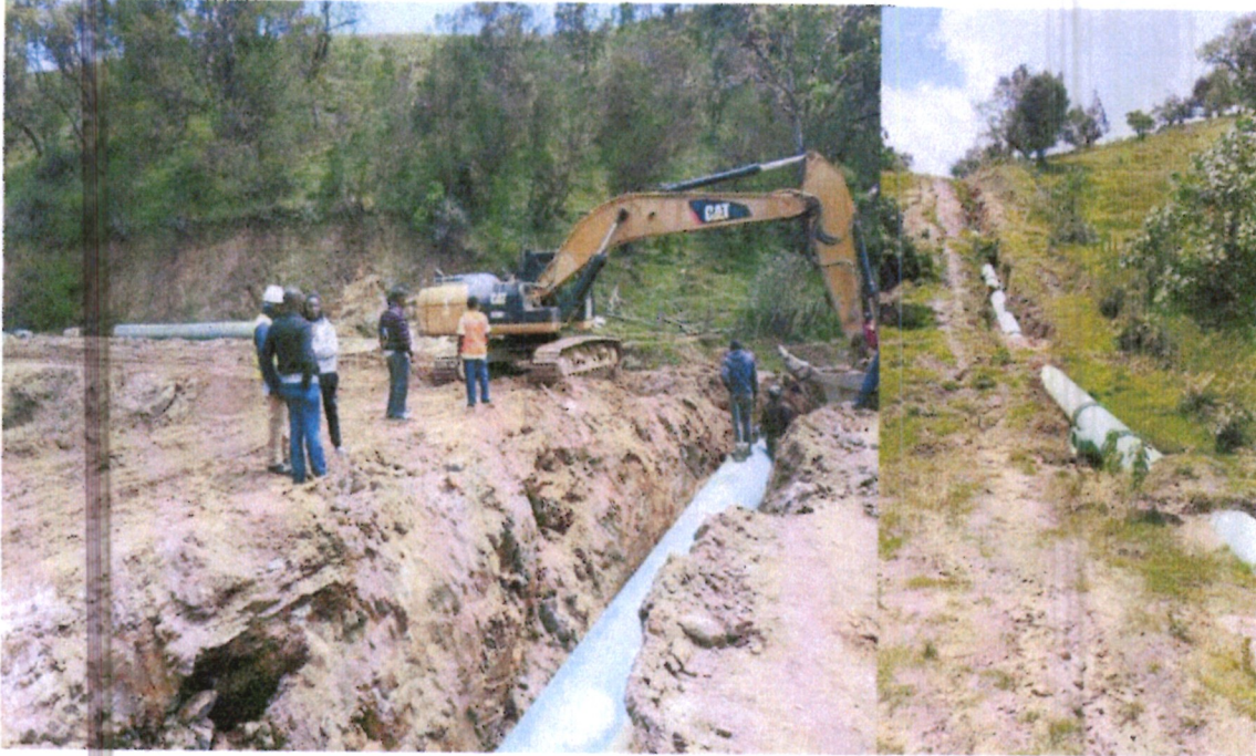
Siyoi (Muruny) Water Supply Projects in West Pokot County and raw water mains pipeline
