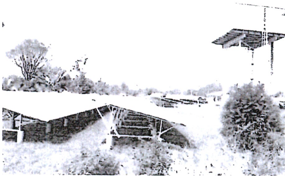
SOLAR TIE GRID SYSTEM- MUNDIKA WATER WORKS
