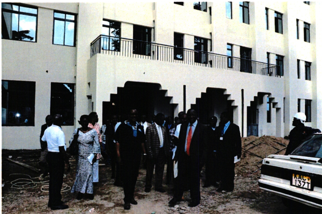
H.E Deputy Governor leads a team of Kenyan ambassadors on a tour for inspection of High Dependency and Intensive Care Unit at Busia County Referral Hospital. Construction ongoing.
