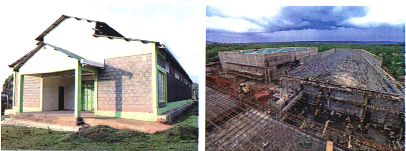
Fig 6. Value addition pack house at Youth Farmers Ongoing construction of Avocado Value Addition Plant
