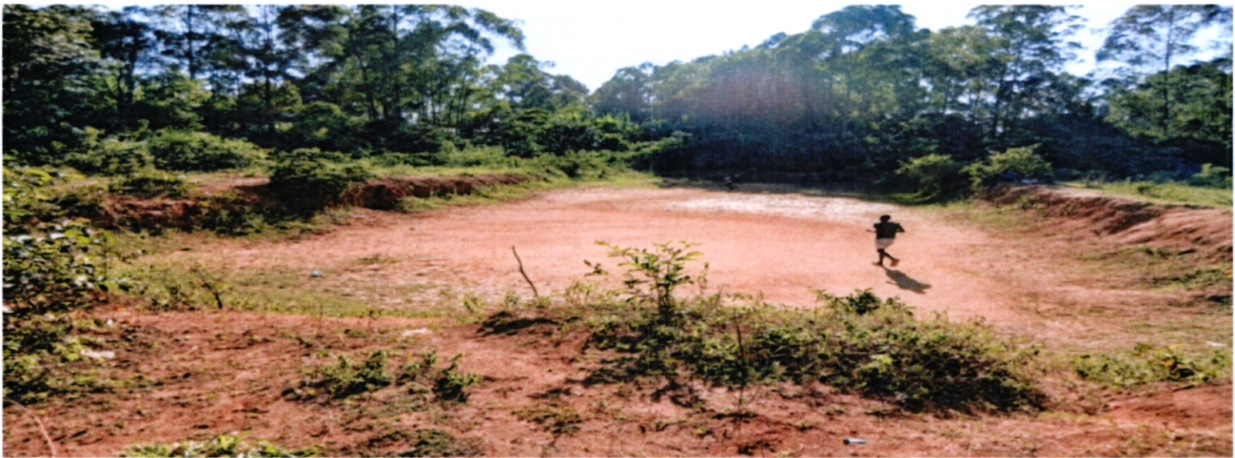
Stalled Sewerage Pond under the Maraba Sewerage Project in Kakamega turned into a playground (photo taken 17 December, 2024 by OAG auditors)
